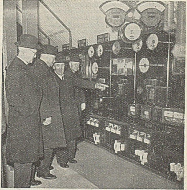
Guests inspecting the switchboard. Left to right: ALD. GILL, chairman of the Electricity Committee, SIR WILLIAM WALKER, ALD. KING, the Mayor, and COUNC. BAKER
