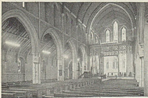
Thirty-four 5 ft. 80 W, Osram "warm-white" fluorescent lamps are used in the lighting scheme just installed at St. Paul's Church, Haringay
