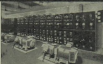
CONTROL in the REFINERY
