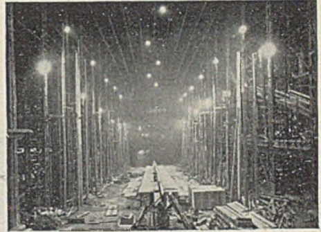
A system of floodlighting installed in a shipbuilding berth
