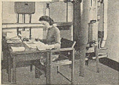
"B. & A." Boiler in leading firm of Dyers & Cleaners.
