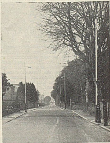
A main street in the Burgh of Cupar, Fifeshire, in which Metrovick "Poplar" lanterns and 140 W sodium discharge lamps have recently been installed. The Metropolitan-Vickers Electrical Co., Ltd., have carried out an extensive modernisation of the street-lighting in the town, using discharge lamps on the main thoroughfares and tungsten lighting elsewhere
