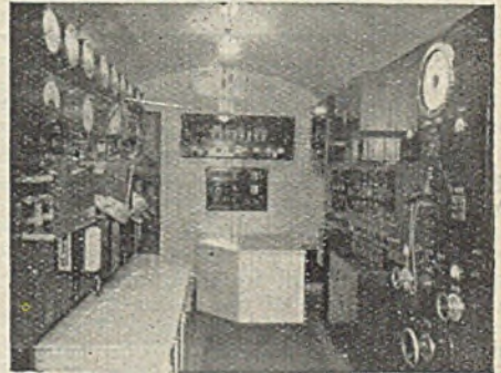
The control compartment, in which the principal controls of each braking unit are centralised
