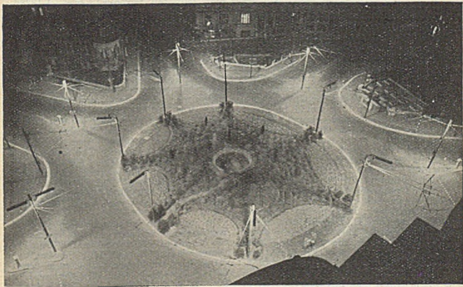
Twenty-five Osram 5 ft. fluorescent tubes in single-lamp cut-off reflector lanterns, providing an average intensity on the roadway of three ft.-candles, make this new installation at the Lansdowne roundabout, Bournemouth, what is believed to be the first of its kind in the country. The lanterns, which are of G.E.C. design, are mounted on brackets on the existing trolley-bus poles. Mr. C. Coffin (public lighting superintendent), under the direction of Mr. W. C. Clowes (borough engineer and surveyor), was responsible for the installation
