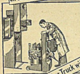
Circuit Breaker being racked down for isolation
