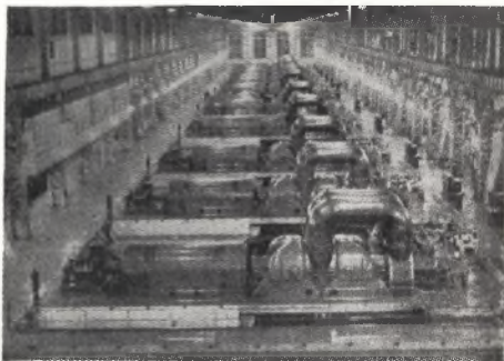
The interior of the Klip station, showing 12 33 MW sets
