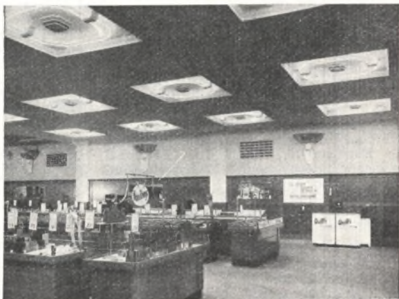
The new fluorescent lighting installation at the Pantheon Store of Marks and Spencer, Ltd., comprises 16 fittings, one in each of 16 panels
