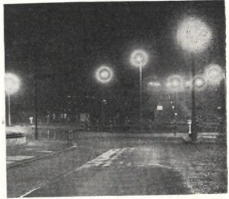
New York Road, Leeds, where 35 G.E.C. h.p.m.v. fluorescent lamps have been installed
