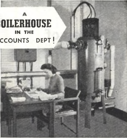
"B. & A." Boiler in leading firm of Dyers & Cleaners.
