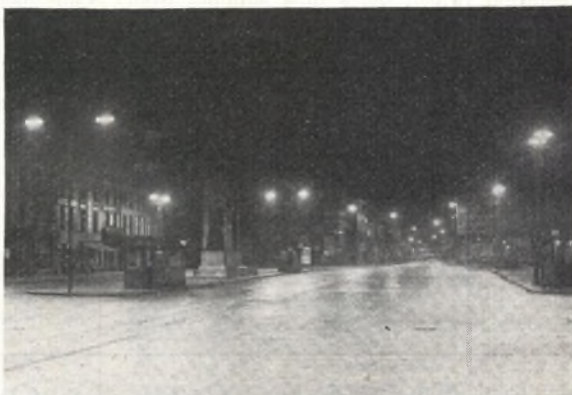
The Revo "blended sodium" lighting installation at Bolton
