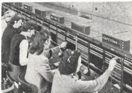
Section of a switchboard at the new Overseas Radio Telephone Exchange. Reduced height affords operators more light and air
