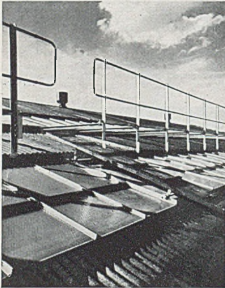
Fig. 4.—Further example of the application of light-metal glazing bars (Westminster Central Depot).
