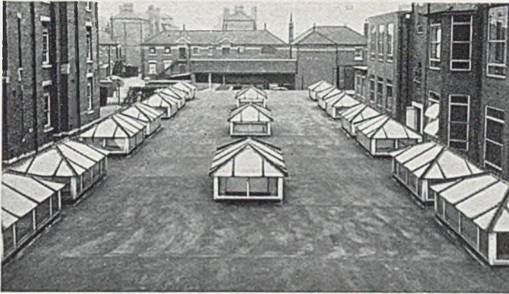
Fig. 1.—View of part of roof of L.C.C. Hospital, Ducane Road, Hammersmith, showing aluminium glazing bars in lantern lights. These bars have been in position for nine years and, although provided with no protective coating of any sort, are still in excellent condition.
