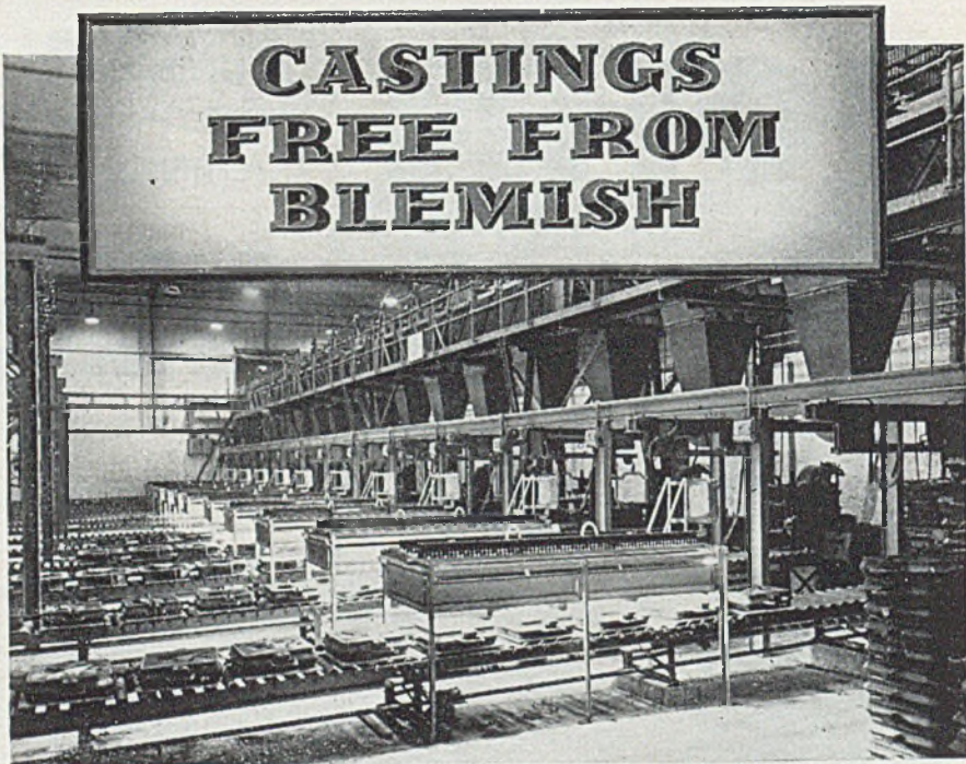
Part of foundry containing 38 Infra-Red units. Loading 342 kW., 1,368 Osram Infra-Red Industrial Lamps.
