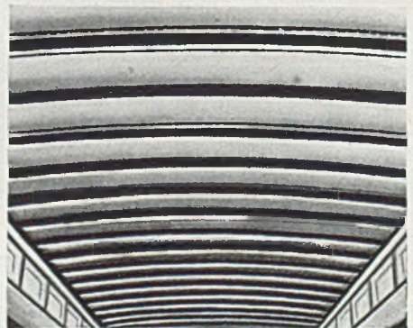
S HOWN in course of construction here is the light-metal roofing for the coaches of the Illinois Central System.
