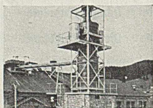
Cottrell Electrical Precipitator collecting sulphuric acid mist at smelter.
