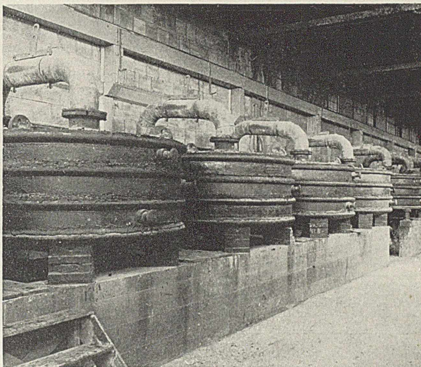
Mineral wool filters for removing impurities out of sulphur dioxide gas in sulphuric acid plant of Ozark Chemical Co.
