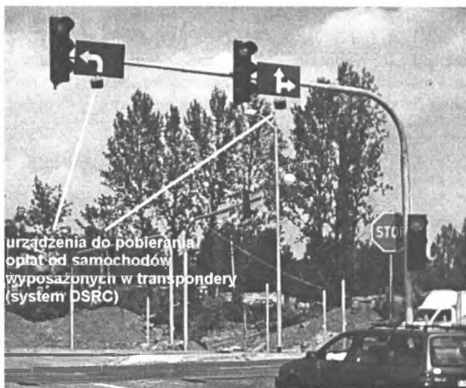
Fig.3. Devices serving the purpose of fee collection in the DSRC system installed on the structure designed to support the light signals [6]
