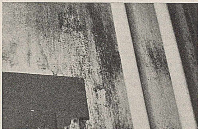
FIGURE 1. MOLD GROWTH ON WALL NEAR REFRIGERATION PIPES
