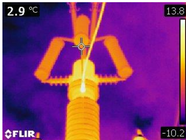
Fig. 4. The thermogram shows the slightly higher temperature for the wire and isolation at the 110 kV voltage side of power transformer (autotransformer: 220/110/15 kV, 160 MVA). The thermogram was made with a FLIR E50 camera
