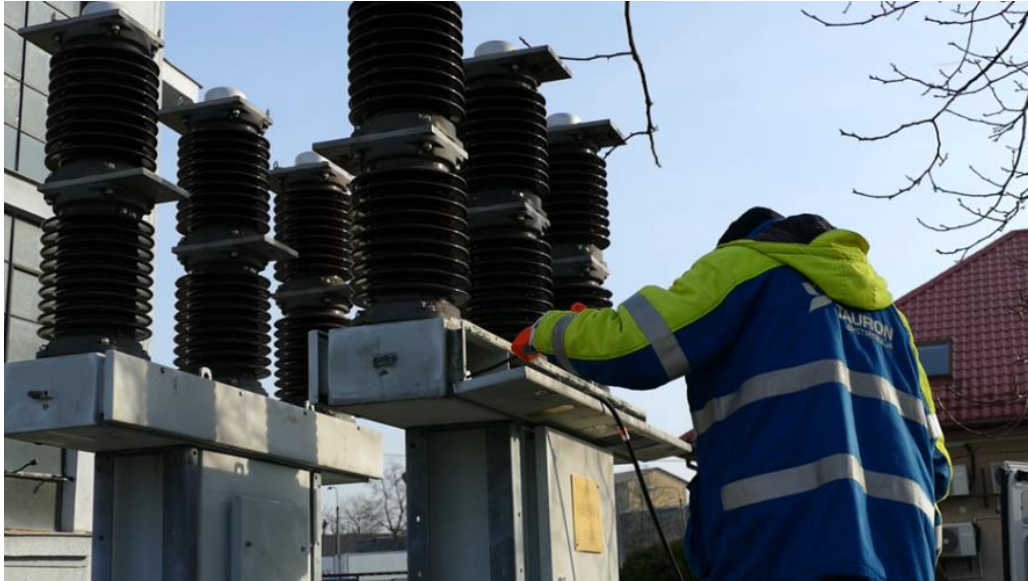
Fig. 7. Testing SF 6 gas leakage from an electric switch, using a chemical detector. (Switch type: ABB OHB 1539; U_N=110 kV), [photo: A. Lisowska-Lis]
