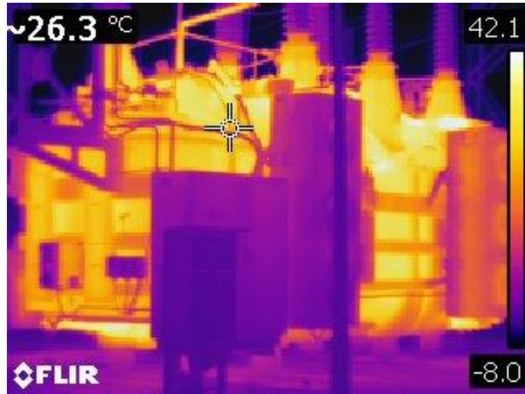
Fig. 2. The thermogram presents transformer with ineffective cooling. The surface temperature is almost even, despite the working fans and cooling circulation (autotransformer: 220/110/15 kV, 160 MVA ). The thermogram was made with a FLIR E50 camera
