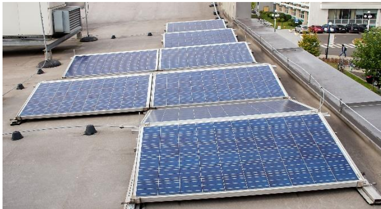
Fig. 5.1 PV array located on the roof of building D4, AGH University of Science and Technolog polycrystalline silicon type.
