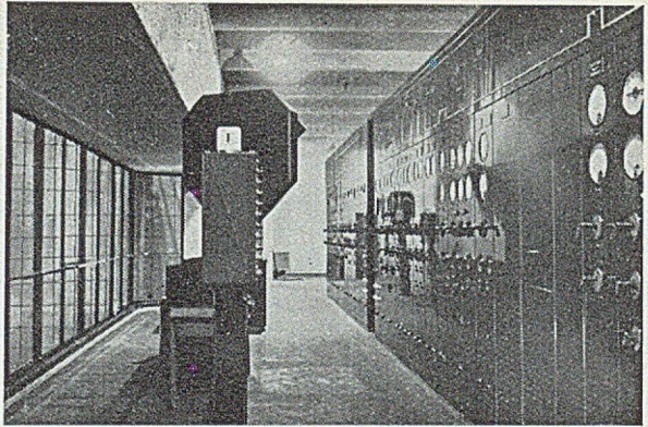
In emergency it has been possible to control both Battersea stations from the emergency control room overlooking the "B" turbine hall
