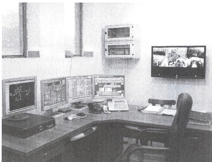
Rys. 13. Stanowisko monitoringu zlokalizowane w rozdzielni Fig. 13. Monitoring stand located in the dispatch and switching station
