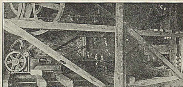
FIG. 4—GENERAL VIEW OF HYDRAULIC PUMP (TO LEFT), ELECTRIC MOTOR (TO RIGHT) AND PULLEY, SPROCKET AND GEAR ARRANGEMENT FOR OPERATING THE PUMP SLOWLY ENOUGH
