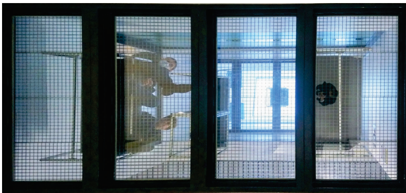
Fig. 42. EHTIC – Glazed shafts providing additional light to the circulation routes and internal rooms. In the picture: a recreational annexe between rooms 102 and 103, on the first floor, seen from the ground floor
