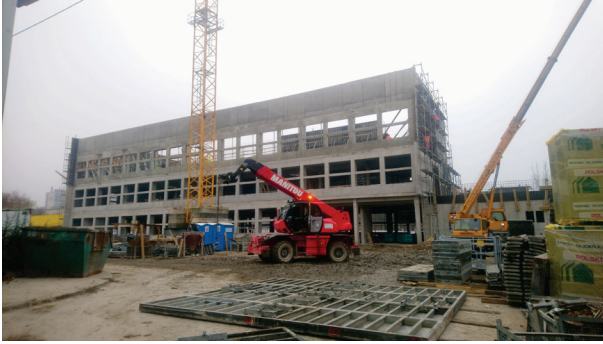
Fig. 10. Construction of the EHTIC edifice. The skeleton of the building - a view from north-west. State of works as of November 2020. Photo by T. Wagner
