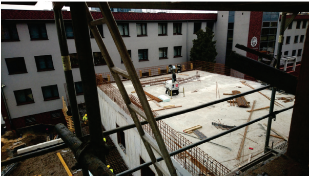
Fig. 12. Construction of the EHTIC edifice. The Philips Auditorium after the installation of hollow-core slabs of the terrace roof. State of works as of the end of November 2020. Photo by T. Wagner
