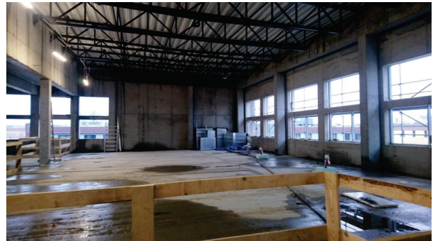
Fig. 13. Construction of the EHTIC edifice. The second floor, the hall of the human motor organ laboratory, after the installation of the truss ceiling. State of works as of January 2021. Photo by T. Wagner
