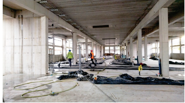
Fig. 11. Construction of the EHTIC edifice. The structure of the ground floor – a view from the space of the main hall. State of works as of December 2020. Photo by T. Wagner
