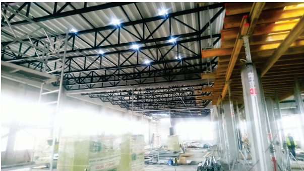
Fig. 14. Construction of the EHTIC edifice. The second floor – roofing over the vast space of the northern belt of laboratories. State of works as of January 2021. Photo by T. Wagner
