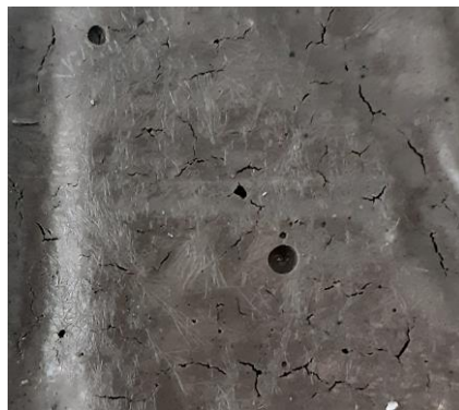
Fig. 12.7. Cracks on the surface of sample from series 8, few minutes after demolding
