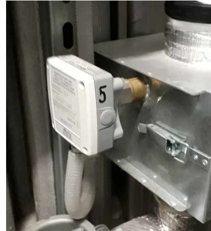
FIGURE 3.5: Air speed and relative humidity transducer mounted in air filter in EM mill installation
