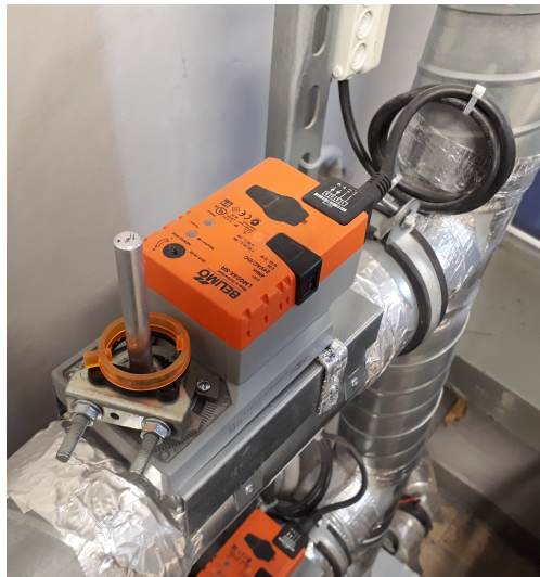
FIGURE 3.3: Electric actuator placed over a butterfly damper in air inlet pipe of EM mill installation
