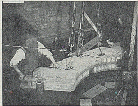
FIG. 30.—Re-assembling one of the Larger Evaporator Bodies. The First Part replaced in position was the Distance-piece which increased the Length between the First and Second Joints.
