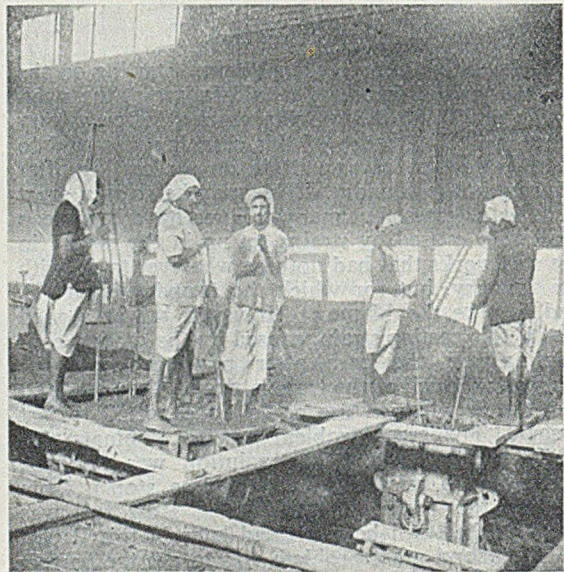
FIG. 2.—A Pit ensures Ease of Ramming, being of such a Depth as to bring the Whole Assembly to Floor Level.
