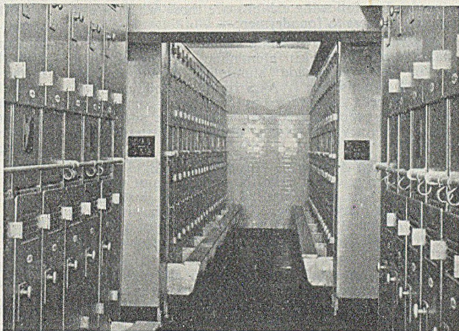
FIGS. 1 TO 4.—Views of the Amenities Block at K. & L. Steelfounders & Engineers, Limited; (top, left) One of the Hand Driers, (right) a Locker Room; (bottom, left) Individual Washbasins and (right) Shower Cubicles.
