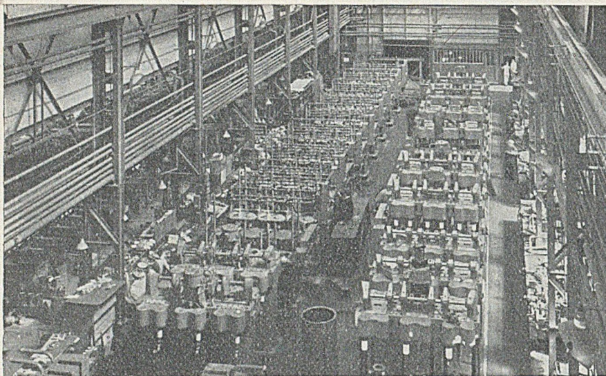
FIG. 10.—General view of one of the Power-station Switchgear Erection Bays at A. Reyrolle & Company, Limited.
