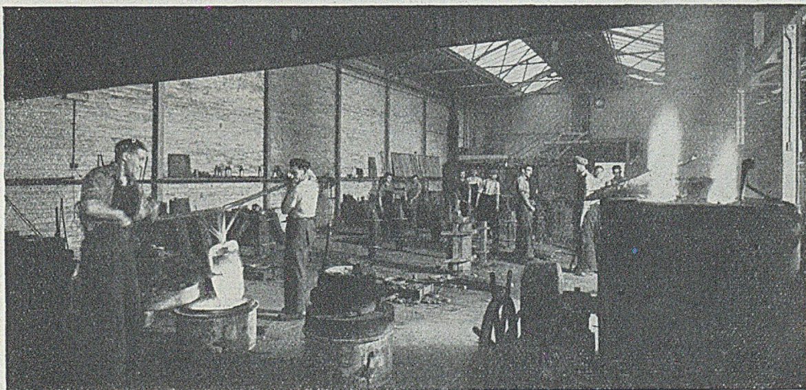
FIG. 4.—Impression gained by looking from the Melting Section, under the "Curtain" to the Chill-cast Bay. The "Curtain," which effectively prevents fumes from spreading, reaches to within 8 ft. of the Concrete Floor.
