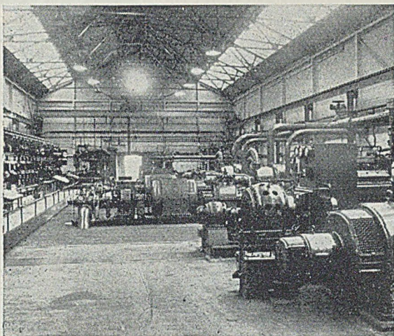
FIG. 4.—General View of the Power Station at Ley's Malleable, where Waste Heat from the Reverberatory Furnaces is Utilized.
