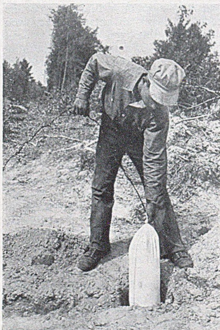
WORKMAN lowering a packaged magnesium anode unit into hole adjacent to pipeline to be protected.
