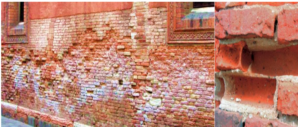
Fot. 3.2-1. Korozja solna muru [W 24], [W 25] Photos 3.2-1. Salt corrosion of masonry [W 24], [W 25]
