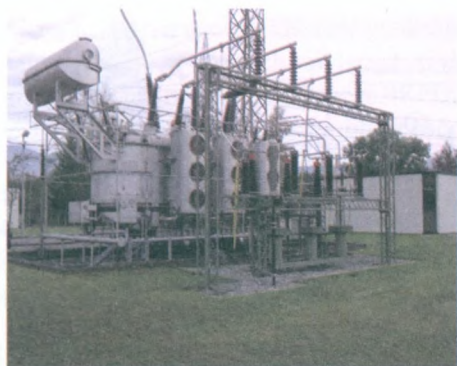
Rys. 1. Transformator 130/130/100 MVA-230/115/48 kV
