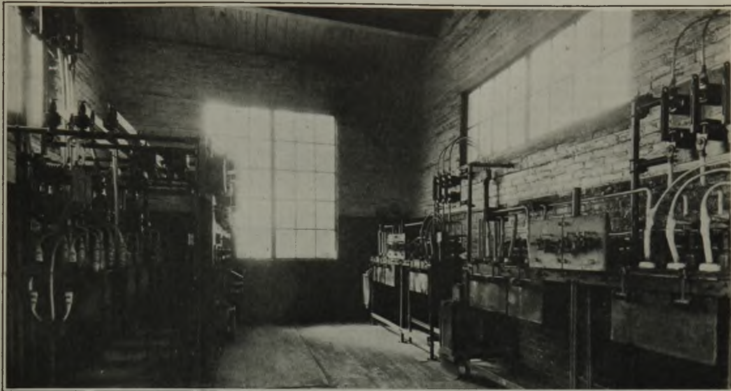
Control House for Substations
