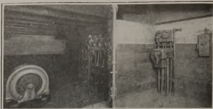
Fig. 8—Control Buttons Outside of Red Ash Bed Substation
