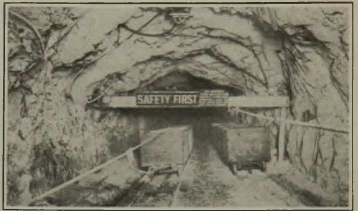
Fig. 3—Improved Lighting Due to Stone Dusting
