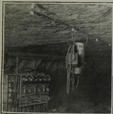
Batteries Are Readily Charged in This Station
