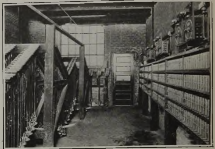
Interior of Lamp-Charging Station
