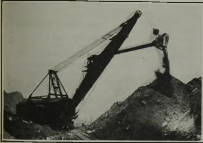
Stripping Coal Electrically at Cuba, Ill.
