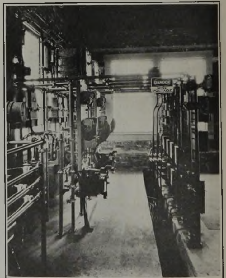
Fig. 4—Back of Main Board, Arcadia Substation
