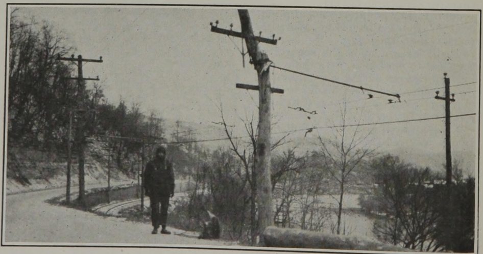
Attempt to Blow Up Western Maryland Ry. Bridge Wrecks High-Tension Pole
