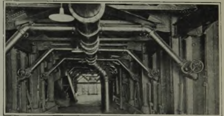
Fig. 8—Piping System Supplying the Jigs
