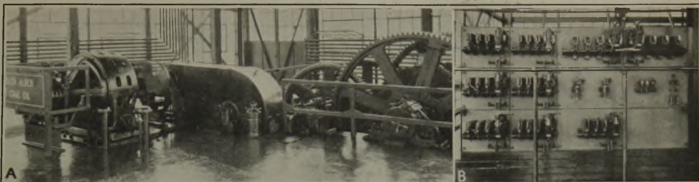
Main-Conveyor Drive and Control Panel, Baker Breaker
