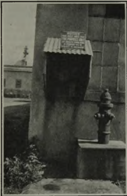
Fire Hose Protected from Weather
