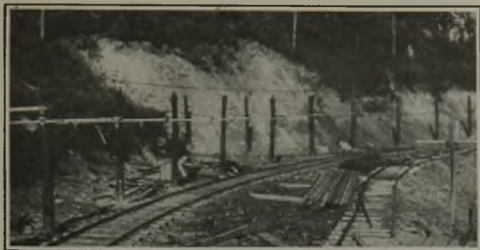
Trolley Supports in Perfect Alignment
