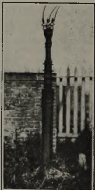
Cable Pot Head A thick coating of pitch covers the pot head on this 2,300-volt armored cable and its junction with the 5 1/2-in. casing.
