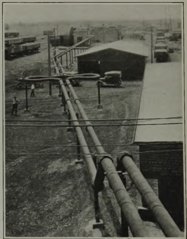
Here Two Fans and Two Steam Lines Guarantee Continuous Ventilation
