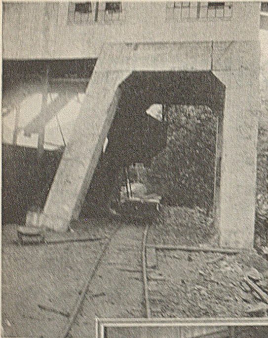
These Columns Supporting the Shaker Drive Are Integral With a 20x24-Ft. Mat, 11½ Ft. Below the Track
