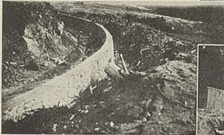
Part of a continuous stretch of 7,800 ft. of wall. There is another section of 1,500 ft. The walls average 6 ft. in height, are 18 in. wide at the top, and have a 3-in.-per-ft. batter.
