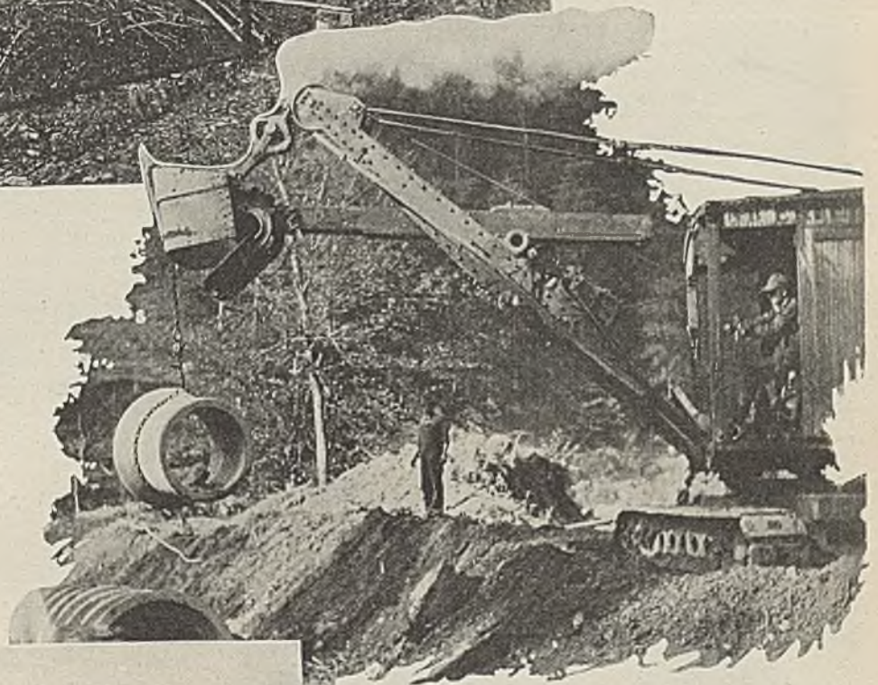
At right—Laying 36-in. reinforced concrete tile in grading the site for yards and town
