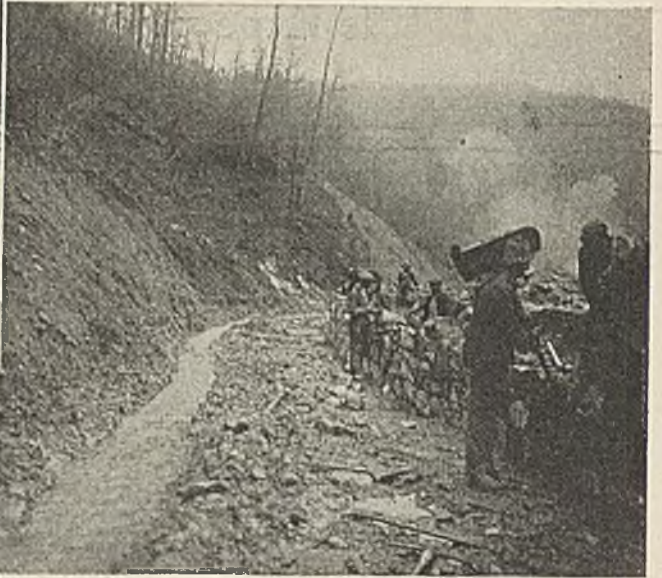
Working on the rubble masonry wall where the creek is to be confined to one side of the valley.
